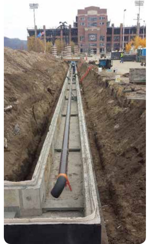
Underground utilities connected the New Student Center into the existing campus utility system.
